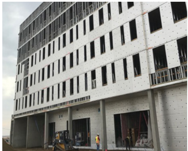
5/8" interior gypsum over steel studs, fiberglass cavity insulation, ECOMAXci® FR, peel and stick WRB. (some areas include metal cladding and 7/8" 3-coat stucco)
