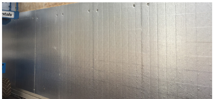
Metal wall panel construction with 8" horizontal metal girt framing, 4" R-13 fiberglass laminated with a vapor barrier and 2" R-13.1 TSX-8500 4x8 insulation.
