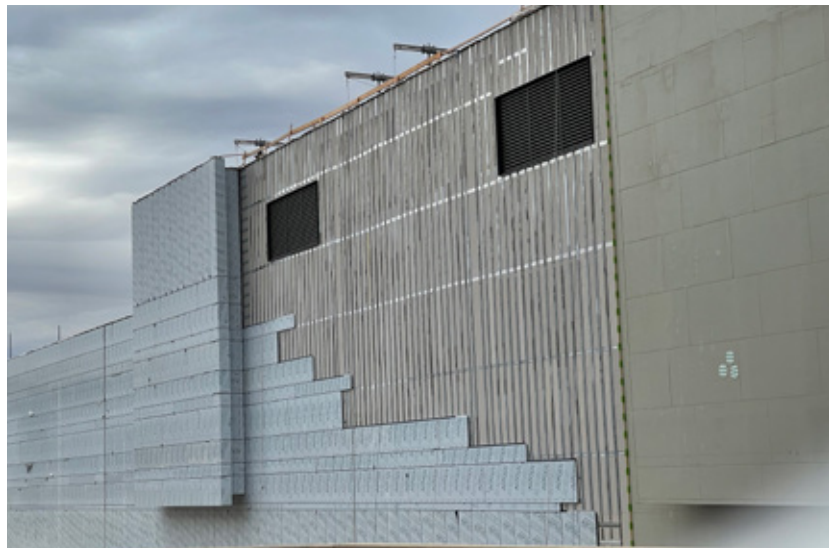
Assembly: Metal studs, exterior gypsum sheathing, air barrier system, Durasheath, ACM panels
